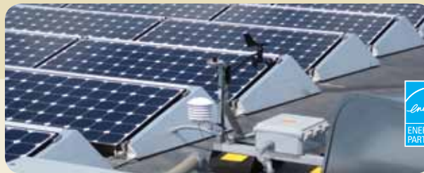
Photovoltaic roof panels, New London, CT branch
